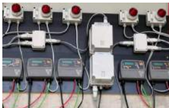
Levels control panel
