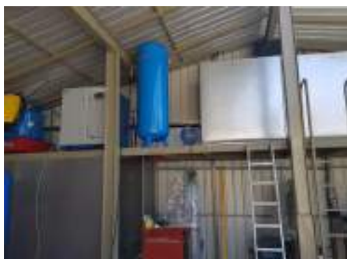
Fluids storage and air-compressor area
