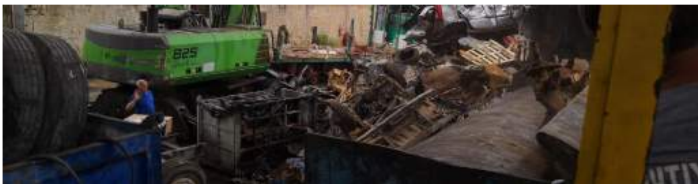
Area of F.lli Montalto before the start of the installation activities of LIFE De-Bay
